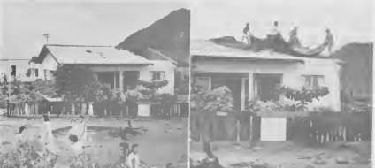
THE STORM seemed to play favorites by leaving some houses completely unroofed, taking whole roofs of others and partially damaging houses such as this one in the Pavilla area.
